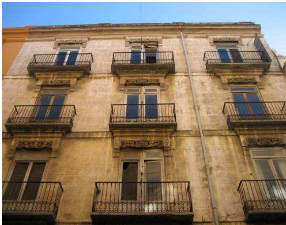
Fig. 1: Façade of a historic building in Valencia's city centre with historic external rendering. V. La Spina.
